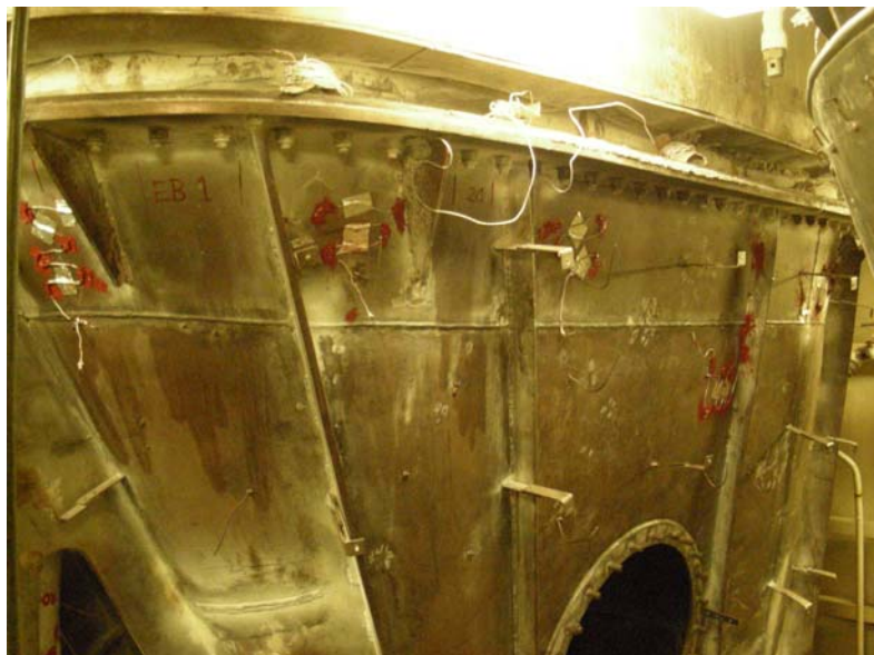
Figure 3. Thermocouples installed in the duct
